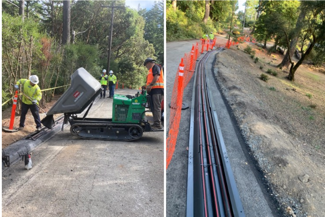
Ground Level Distribution Systems (GLDS) Neither Overhead nor Underground, PG&E Pilot Program Evaluates the Benefits of Putting Powerlines Right on the Ground
